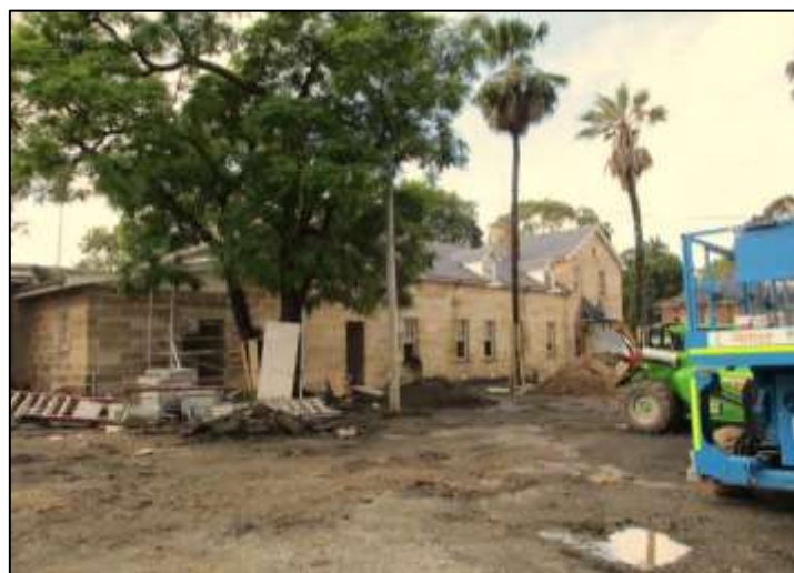
Current construction at the Female Factory site - the Greenway Hospital. Photograph courtesy: Judith Dunn
